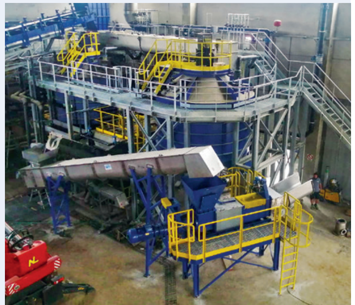
BTA® Hydromechanical Pre-Treatment Castelleone as seen during installation
