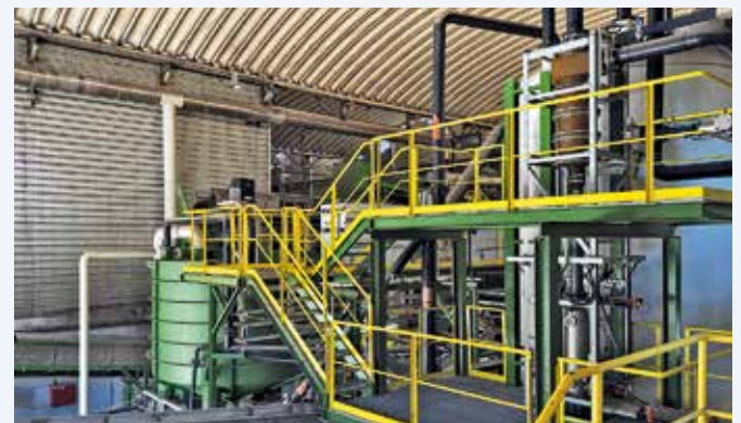
3 rd BTA pre-treatment line in Valorlis
